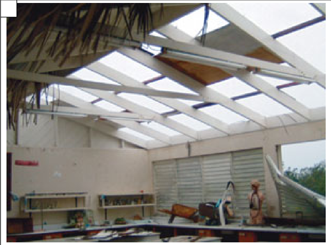
Classroom after the hurricane
